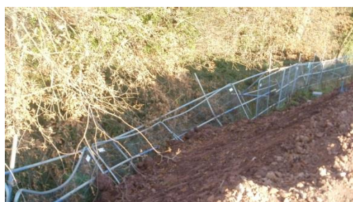
Here, fencing hasn't been secured and has been pushed over by the adjacent soil - this is not acceptable.
